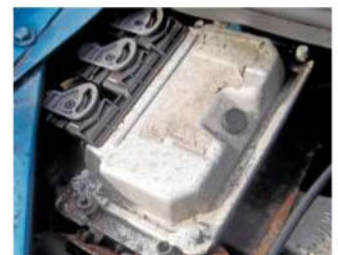
The corrosion had crept into the connecting plugs, resulting in the running problems.
